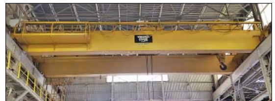
75 Ton/ 30 Ton x 60' Span Virginia Overhead Bridge Crane
