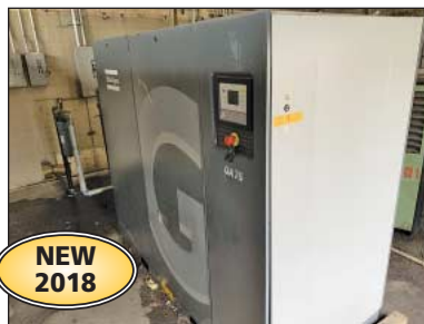
100 HP Atlas Copco Model GA75 Air Compressor
