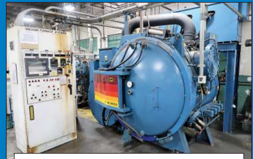
Complete Heat Treat Department
