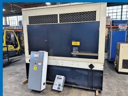
(3) Kohler Diesel Backup Generators
