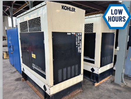
(2) 34 KW Kohler 30RE0ZJB Diesel Backup Generators
