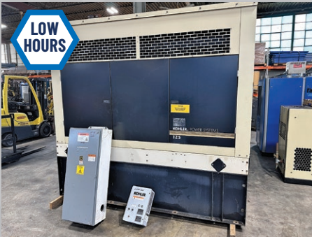
130 KW Kohler 125RE0ZJB Diesel Backup Generator
