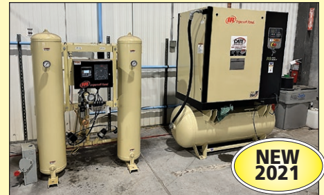
30 HP Ingersoll Rand Air Compressor & Dryer
