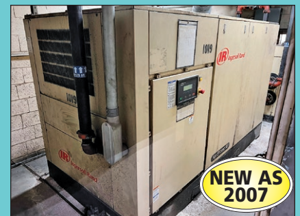
(2) 200 HP Ingersoll Rand Model SSR-EPE200-2S Air Compressors
