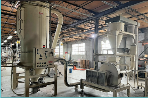
40 HP MAC Pulverizer w/ Cyclone Dust Collector & Mac Hopper
