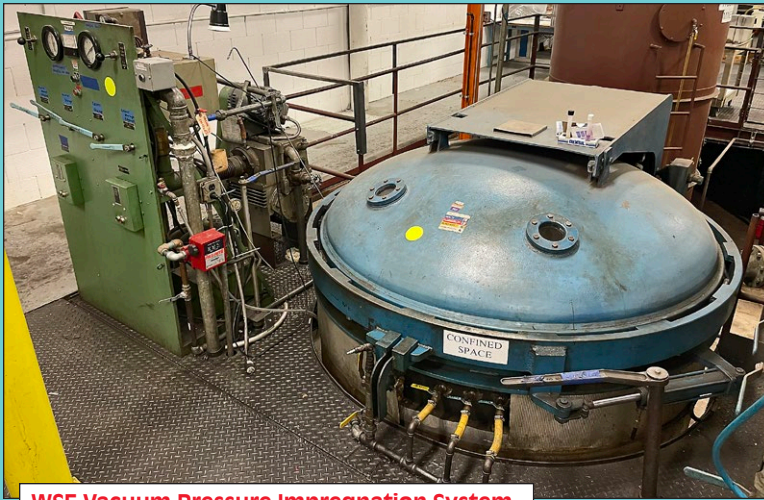
WSF Vacuum Pressure Impregnation System
