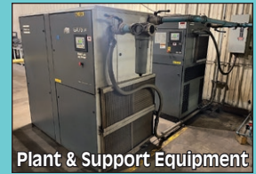
Plant & Support Equipment
