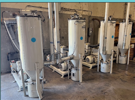
(4) 25 HP Unadyne Vacuum Pumps for Blending Systems
