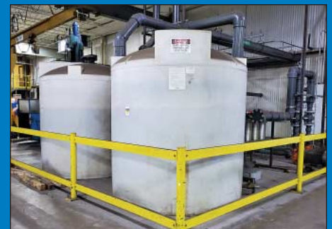
(2) Poly Tanks, Pumps, and Heat Exchangers
