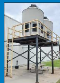
(2) Delta Model T-1251 Fiberglass Induced Draft Cooling Towers
