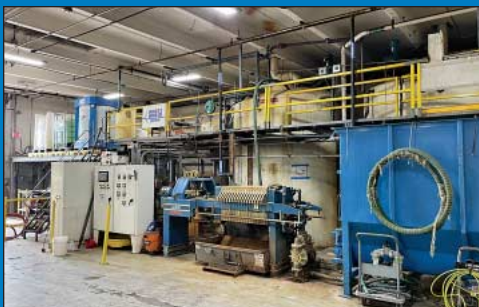
Wastewater Treatment System
