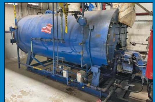
Industrial Boiler Company Model EFDL 125 CG02 Boiler
