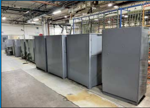
(12) Controlled Power Company RXPO Series 30 Power Supply/Rectifiers
