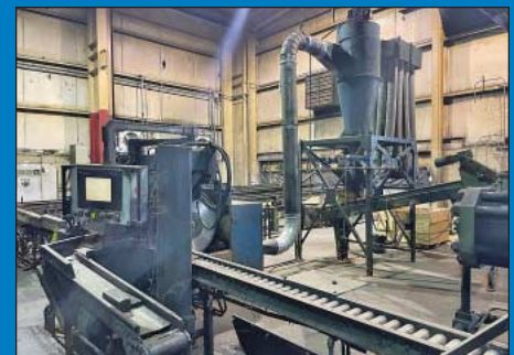
(3) 30" Dia. B&O Automatic Billet Saws w/ Dust Collectors
