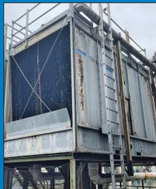
(7) Various Size Cooling Towers by Evapco and Marley
