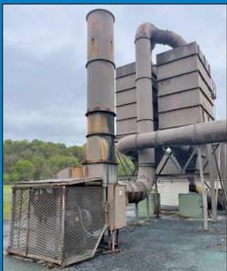
150-HP Wheelabrator Bag House Dust Collector & Blower
