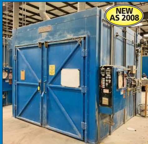
(17) Wisconsin Natural Gas & Electric Batch Ovens
