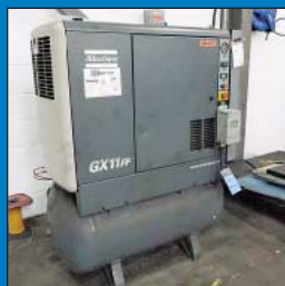
15 HP Atlas Copco Model GX11 Horizontal Tank Mounted Air Compressor
