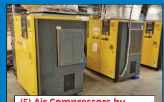
(5) Air Compressors by Kaeser and IR to 25-HP (to 2015)
