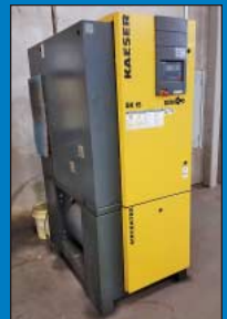
15 HP Kaeser Aircenter SK15 Air Compressor
