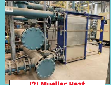
(2) Mueller Heat Exchangers (2007)
