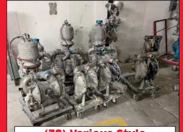
(30) Various Style Stainless Pumps
