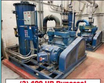
(2) 100 HP Dynaseal Travaini Vacuum Pumps
