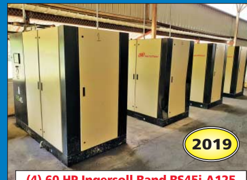
(4) 60 HP Ingersoll Rand RS45i-A125 Air Compressors, Low Hours
