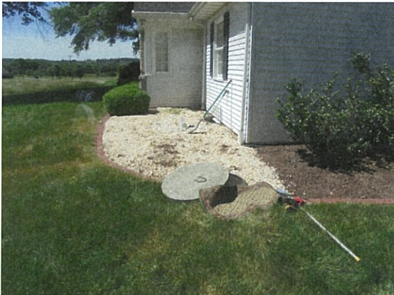
Location of second tank
