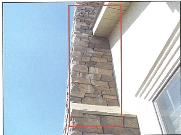
3.0 Item 4(Picture) Efflorescence noted on dry stack veneer, some stone were loose
