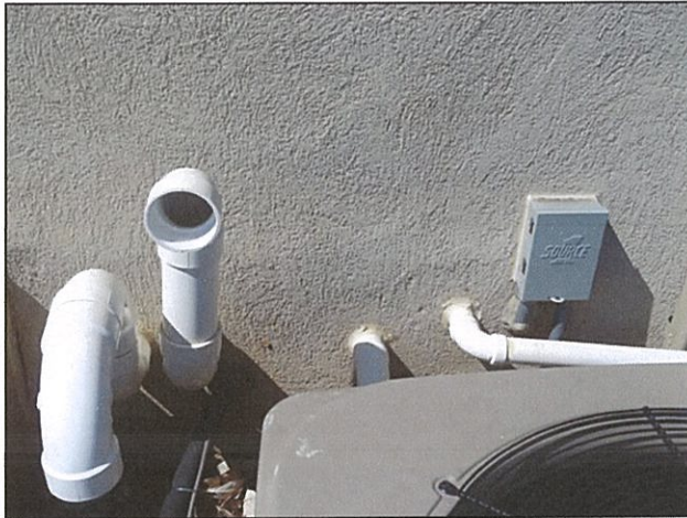
3.0 Item 19(Picture) No flashing boxes were installed on exterior penetrations
