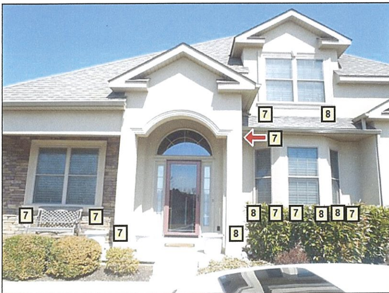
2.1 Item 2(Picture) Left front moisture readings
