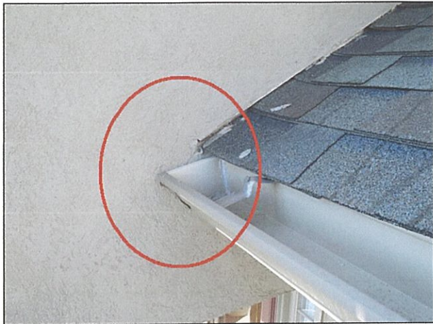
3.0 Item 9(Picture) No kickout flashing installed at roof/wall intersection to right of main front entry. Moisture reading below was 7%
