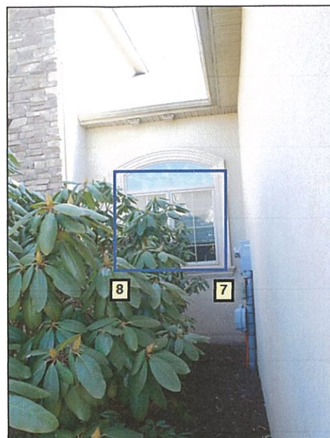
2.3 Item 2(Picture) Rear bathroom window b moisture readings behind garage
