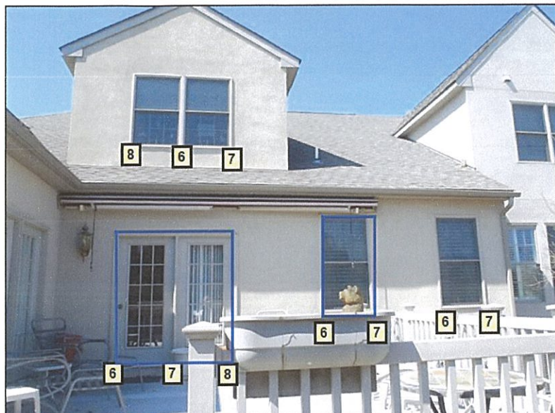
2.2 Item 3(Picture) Right elevation deck entry moisture readings
