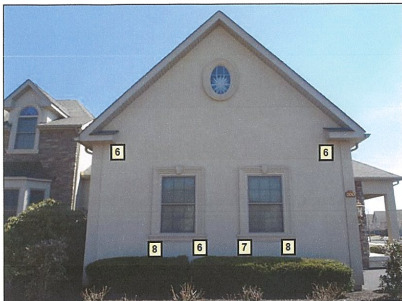
2.3 Item 1(Picture) Left elevation garage moisture readings
