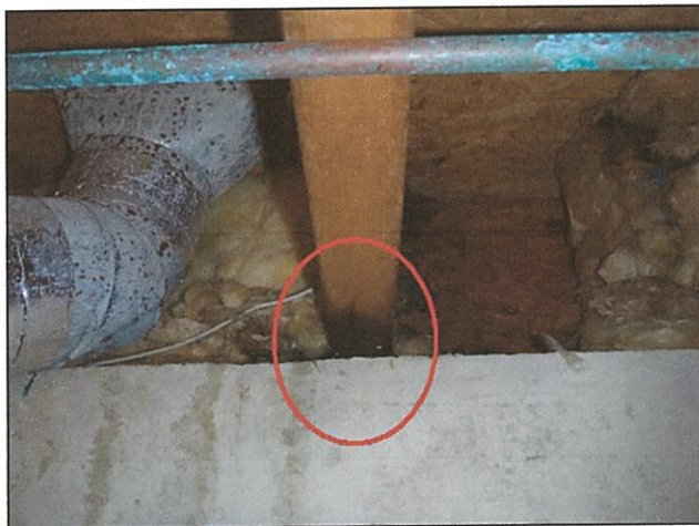
3.0 Item 3(Picture) Moisture intrusion noted on TGI in basement under sunroom entry
