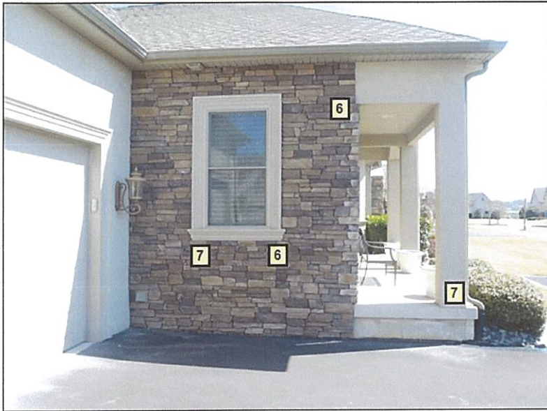
2.1 Item 3(Picture) Left side of front porch, efflorescence noted on veneer
