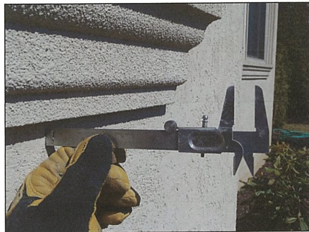
3.0 Item 12(Picture) Stucco measured 1/2" thick in most locations
