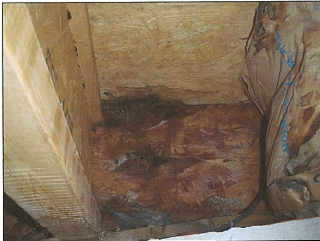
3.0 Item 2(Picture) Moisture intrusion under sunroom doors in basement box beam
