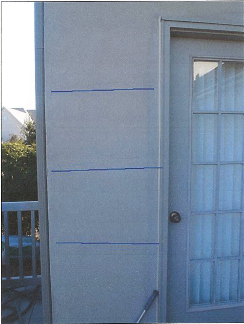
3.0 Item 15(Picture) Multiple cracks noted on left and right side of sunroom deck entry door
