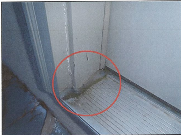
3.0 Item 16(Picture) Moisture damage and heavy sealant on sunroom deck entry door
