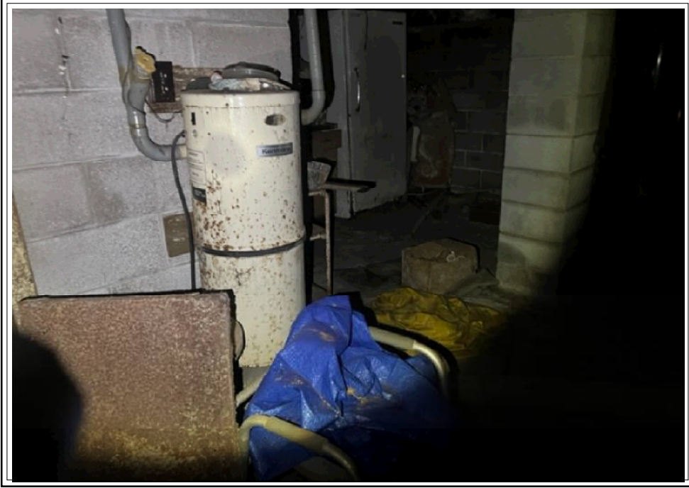
SUBJECT BASEMENT CENTRAL VACUUM PHOTO DATE 10/26/2023
