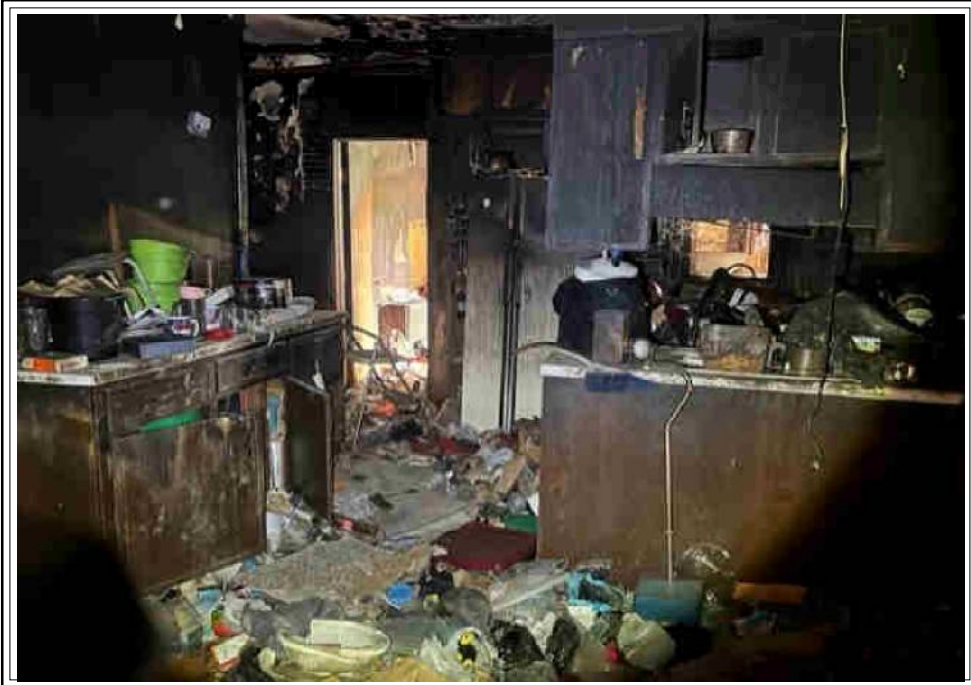
SUBJECT FIRST FLOOR KITCHEN AFTER FIRE PHOTO DATE 10/26/2023
