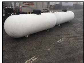
2 - 500 Gallon Propane T4-8
