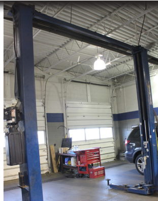
#258 - 273 Challenger, Forward, & Workhorse Automotive Lifts
