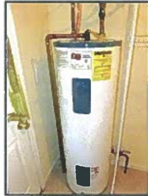
1225 Norfolk Water Heater
