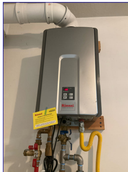
The Water Heater Area
