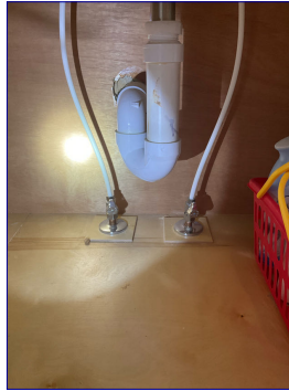
The bathroom plumbing view.
