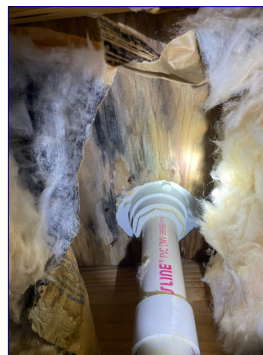
Moisture stains beneath the master shower
