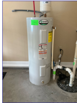
The Water Heater Area
