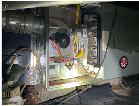
The furnace, cover off
