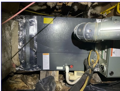
The evaporator coil cabinet
