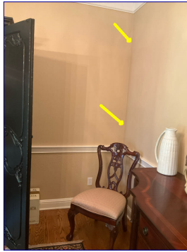
Cracks and wrinkled wallpaper
