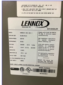
The furnace, data tag
