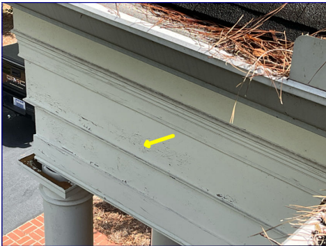
Needs to be scraped and repainted
