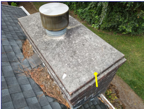
Cracked chimney cap
