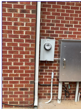
The electrical service drop
