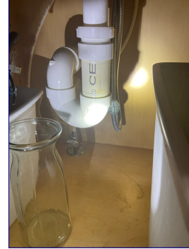
Laundry room plumbing view
