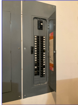
The main electrical service panel (Right)
