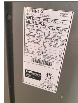
The air conditioner compressor/condenser data plate.
