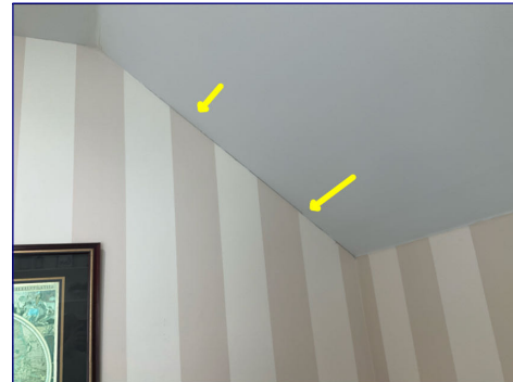
Signs of settling
