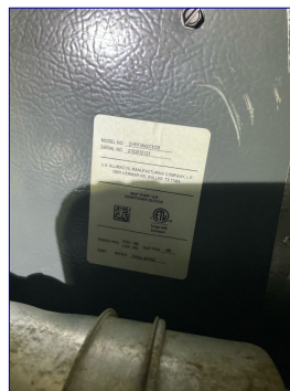
The air conditioner coils data plate
