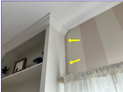
Signs of settling
