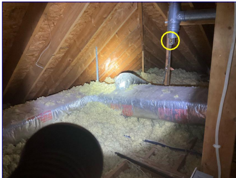
Open junction box
