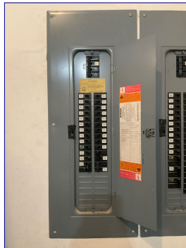
The main electrical service panel (Left)
