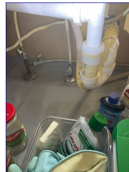
Kitchen plumbing view
