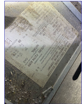
The furnace, data tag
