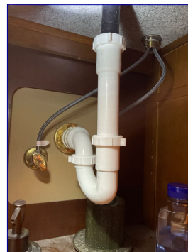
The bathroom plumbing view.
