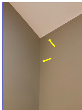
Loose tape seems and settling cracks
