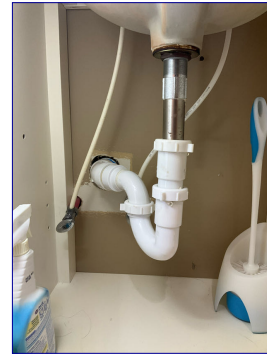
The bathroom plumbing view.
