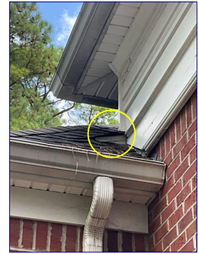
Roof junction above the water stains/damage in the garage
