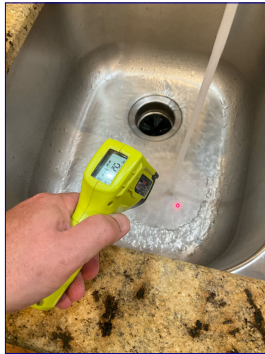
Hot water temp
