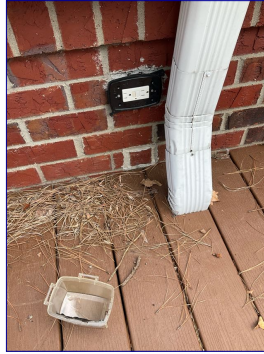
Broken weather cover
