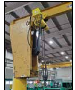
SPANCO 1.5-Ton Jib Crane
