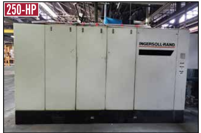
INGERSOLL-RAND 250-HP Rotary Screw Air Compressor
