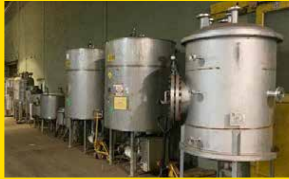
RAS Process Alloy-20 Reactors
