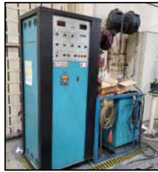
HI-POTRONICS Transformer Unit
