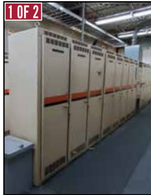
RELIANCE ELECTRIC Engineered VS Drive Unit
