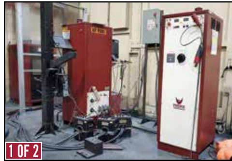
SEISMIC & PHENIX Motor Test Stands
