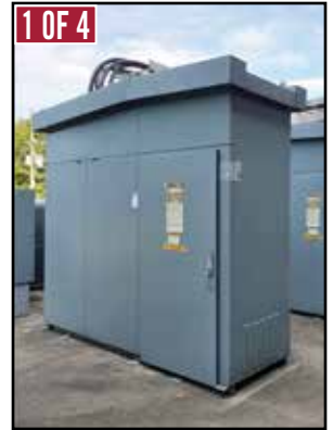
SQUARE D Primary & Secondary Disconnects
